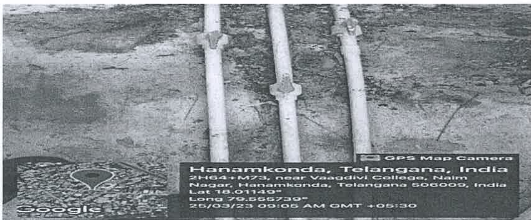
Water Distribution Systems in the College from the Tanks
